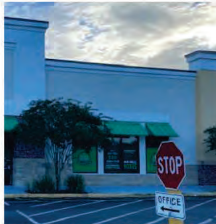
*EXISTING STORAGE SHOP VINYL TO BE REMOVED; SURFACE TO BE CLEANED FREE OF ADHESIVE
