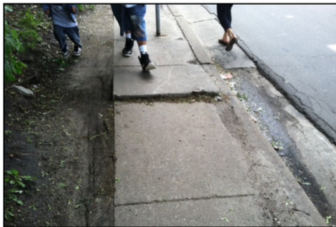
Image of a heaved sidewalk from the Department of Transportation
