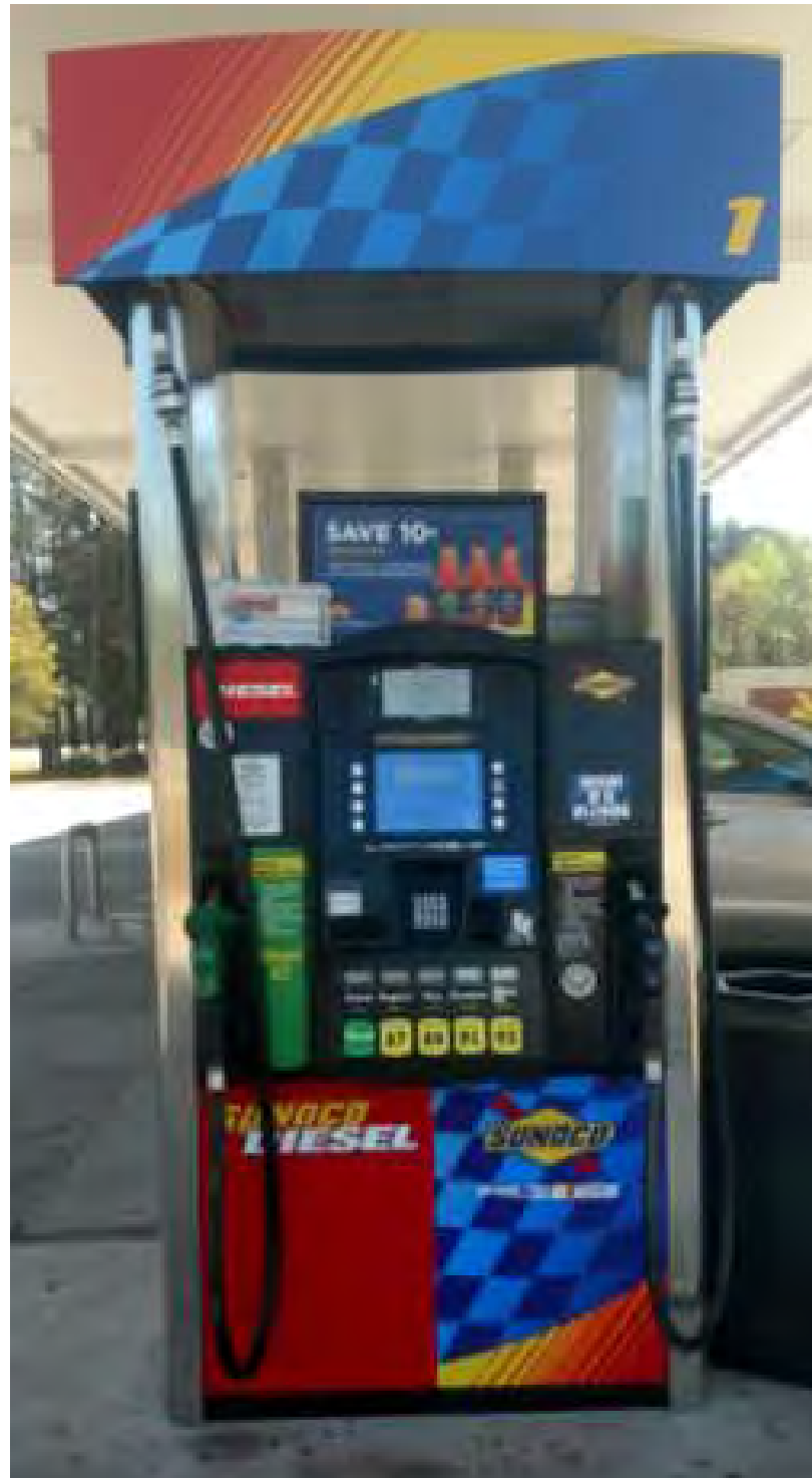
EXISTING FUEL DISPENSERS (6) TYP.
